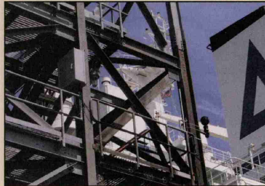
Heavy duty cameras at terminals can communicate via wireless. The key to the Alabama installation is an appliance that allows myriad agencies assigned to protect the supply chain to see what they specifically need in their format.
